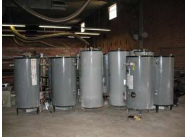
Warehouse 03/06/08 Failed hot water heaters due to scaling
