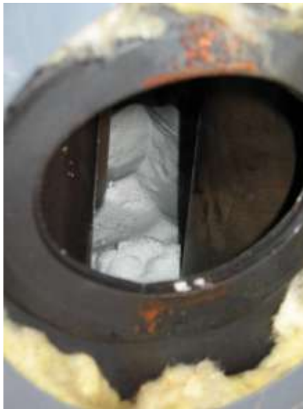
Installed 02/21/07 – room #27 still in service
