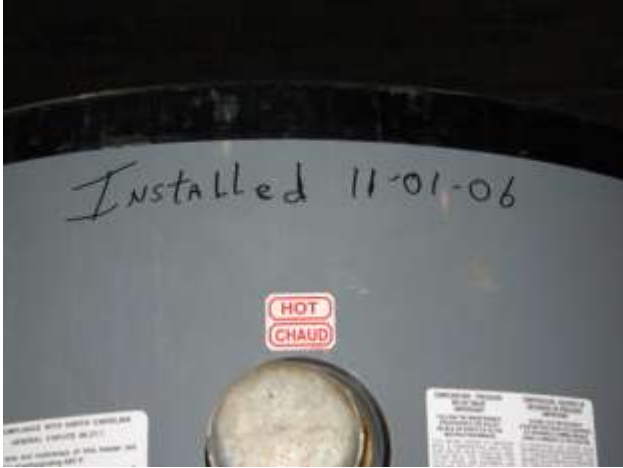
Installed 11/01/06 – room # 1 Failed 02/04/08
